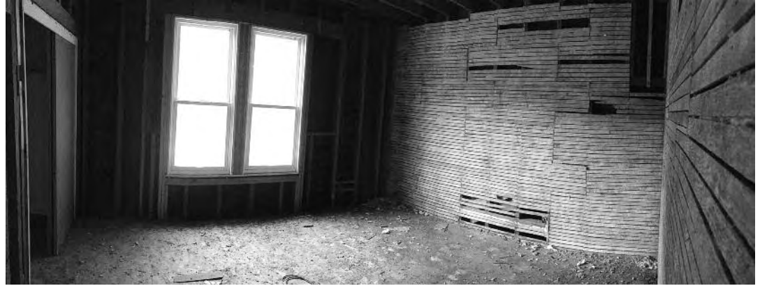
Severely damaged second-floor room in the Faria House.
