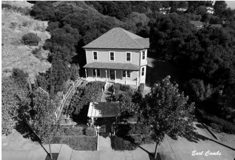
The Faria House sits empty, and deteriorating in Heritage Park on San Pablo Avenue.
